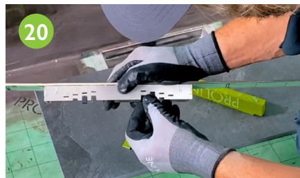
20 Insert the height distance clips in the cascade adjustment of the shower profile frame. The clips are inserted in the respective recesses based on the calculated tile height plus addition of the adhesive bed thickness. Heights between 10 and 17 mm can be realised.
