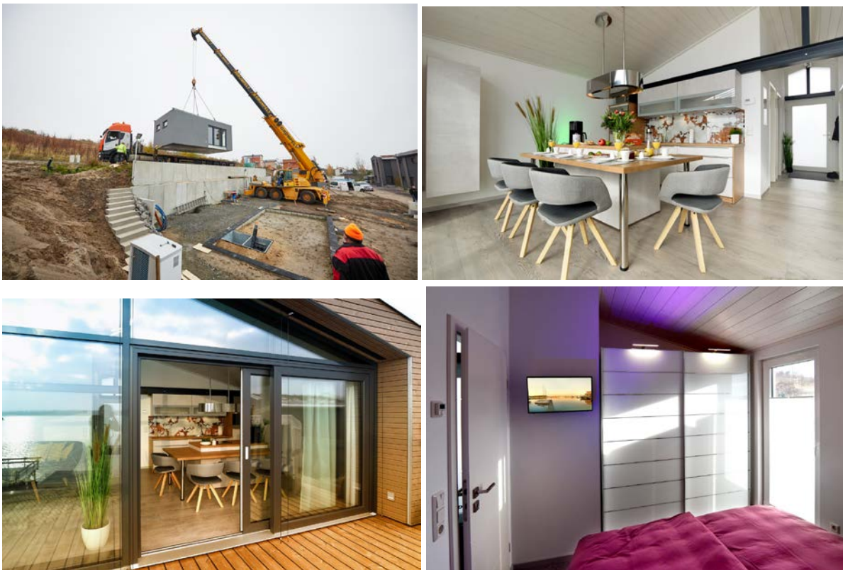
Caption: Laying of the foundation stone, topping-out ceremony and moving in – all on the same day - the Petit Chalet
